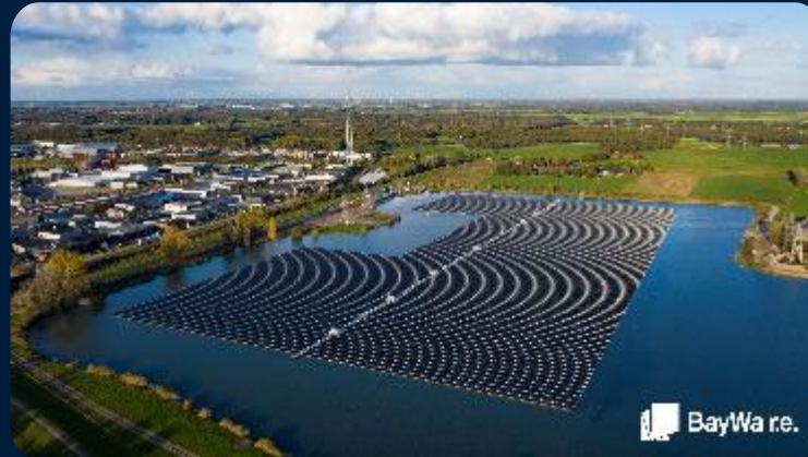
BayWa, Netherlands 27 MW
