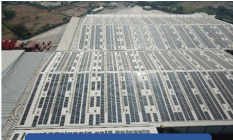
Solar PV rooftop
