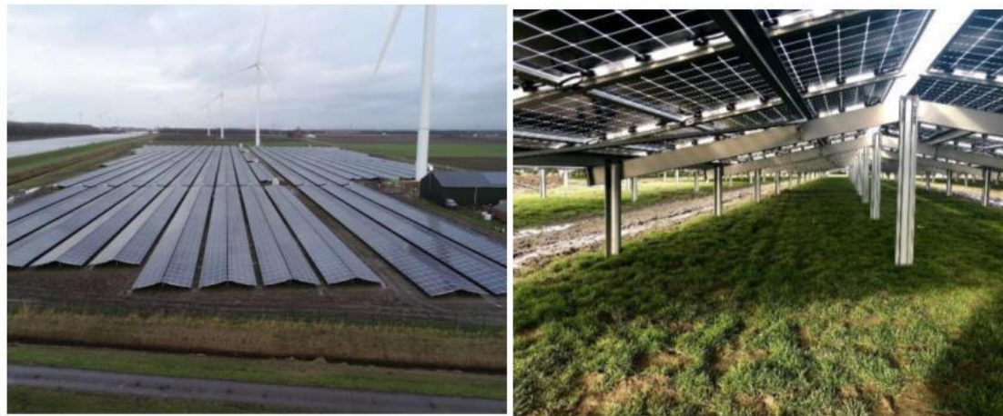
Netherland Zonnepark Rilland 11.75 MW
